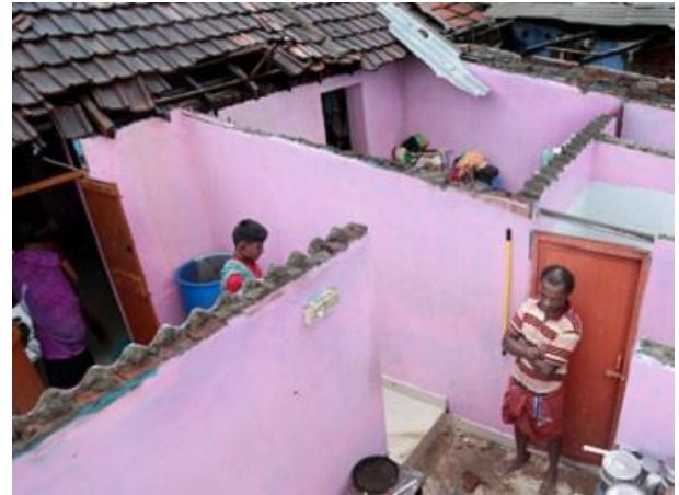
Fig 9. Cyclone Ockhi damaged house in Kanyakumari. courtesy: www.firstpost.Com
